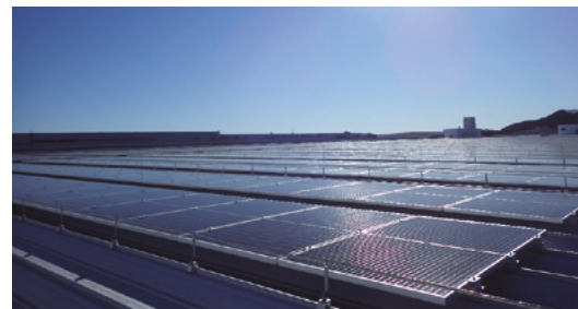
Saitama Factory's Yorii assembly plant (2.0 MW)
